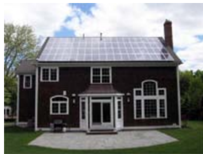
Domestic rooftop photovoltaic system
